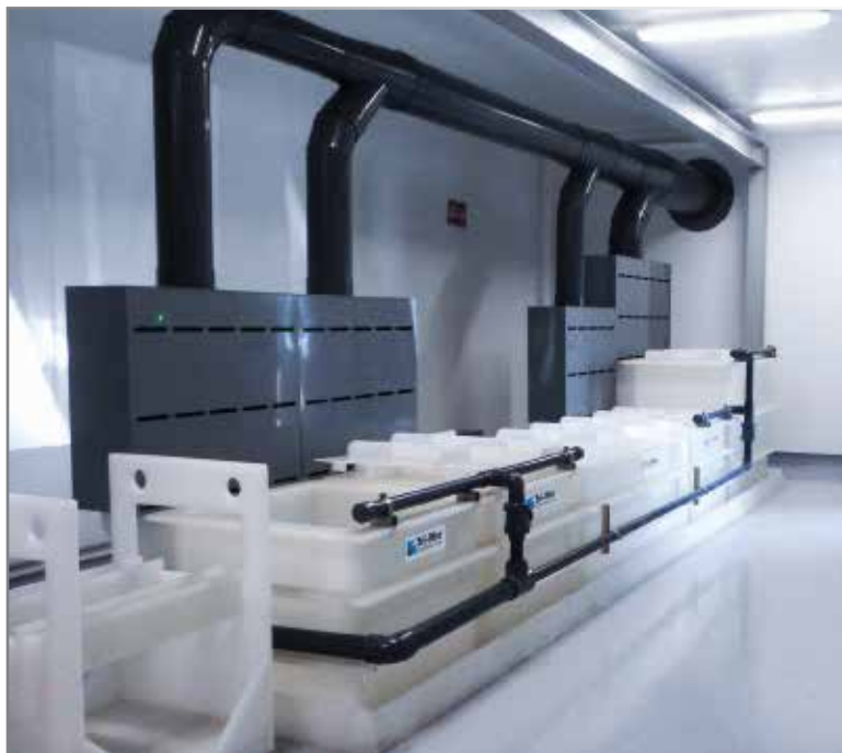
Lateral exhaust via backdraft hood with push air header opposite the hood. All photos: Tri-Mer Corporation.
