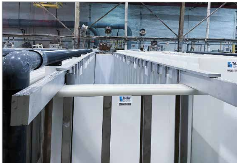
Bottom side lateral (BSL) hood with push air header on anodizing process for architectural extrusions.
